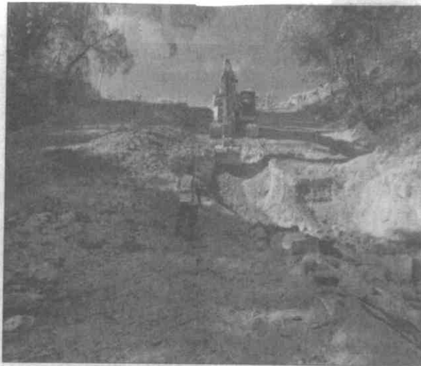
Photos courtesy of El Dorado County Department of Transportation Construction crews build a rock-lined ditch on the south side of the new crossing between Placerville and Mosquito.
